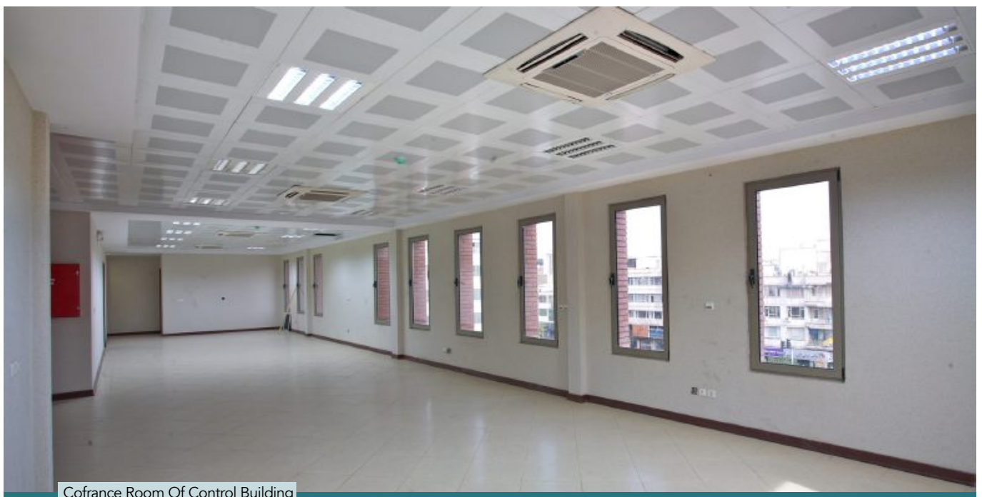
Cofrance Room Of Control Building
