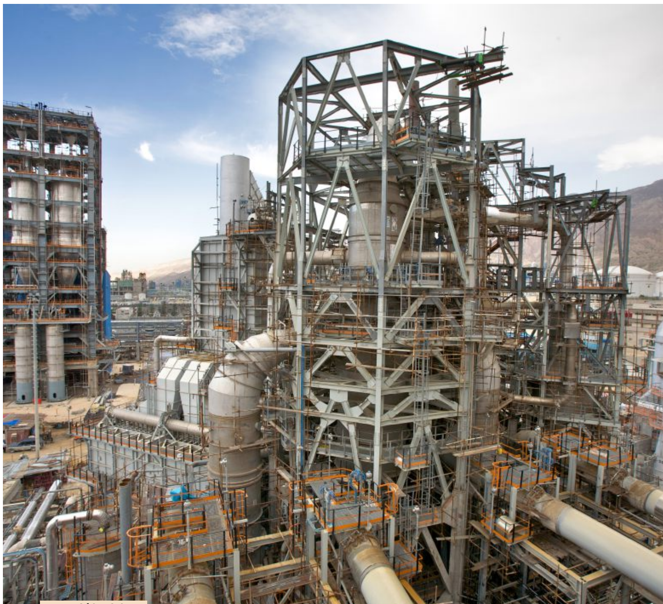
A View Of STRO 2 Unit
