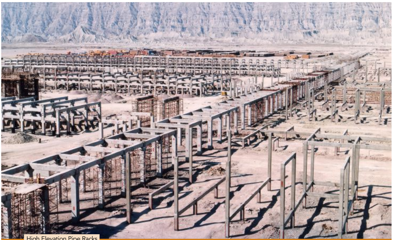
High Elevation Pipe Racks
